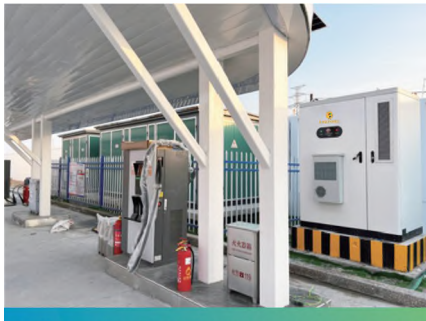
Xinjiang · Electric Vehicle Solar-Storage-Charging Project Scale:100kW / 215kWh
