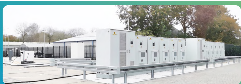
Netherlands · Logistics Fleet Integrated Solar-Storage-Charging Project Scale:1.5MW / 3.2MWh
