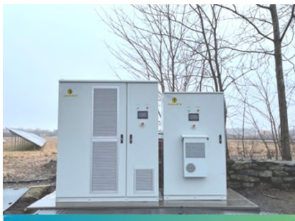
Sweden · Rural Church and Residential Solar-Plus-Storage Solution Scale:125kW / 215kWh
