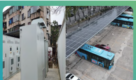
Guilin, Guangxi · Electric Bus Solar-Storage-Charging Project Scale:500kW / 996kWh
