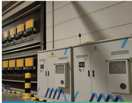
Belgium · Chocolate Factory Energy Storage Backup Solution Scale:350kW / 748kWh
