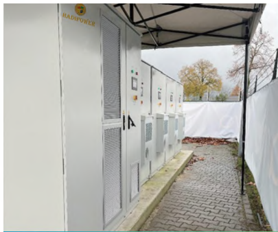
Sweden · Electric Bus Storage-Charging Project Scale:250kW / 860kWh
