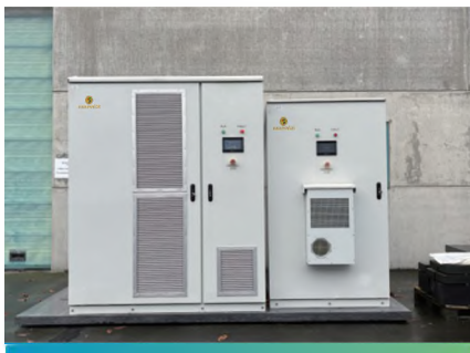
Belgium · Industrial Plant Energy Storage System Scale:100kW / 215kWh
