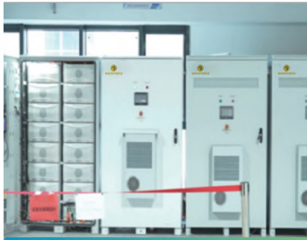
Xiamen · Energy Storage and Backup Power Project for Power Plants Scale:500kW / 1129kWh
