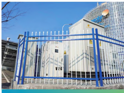
Yiwu, Zhejiang · Commercial Center Solar-Storage-Charging Project Scale:250kW / 215kWh
