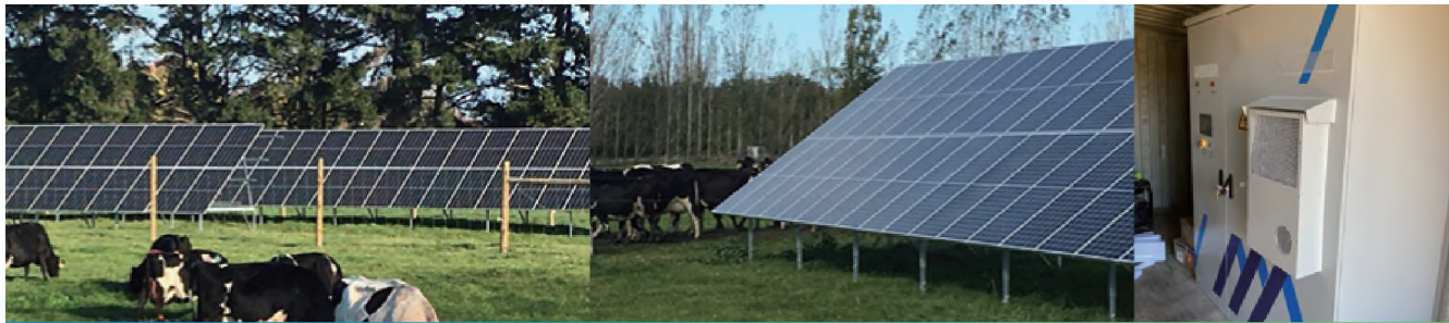
New Zealand · Solar Microgrid Project for Dairy Farm Scale:60kW / 122.88kWh
