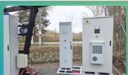
Romania · Integrated Emergency Backup Power and EV Solar-Storage-Charging Project Scale:100kW / 215kWh
