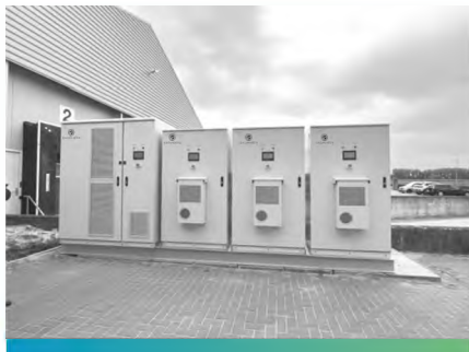
Netherlands · Jam Factory PV-Storage Project Scale:250kW / 645kWh
