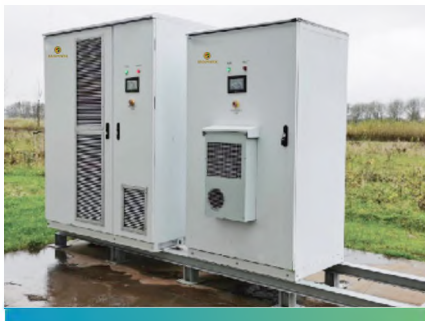
Netherlands · Metal Recycling Plant Solar-Storage-Charging Project Scale:62.5kW / 215kWh
