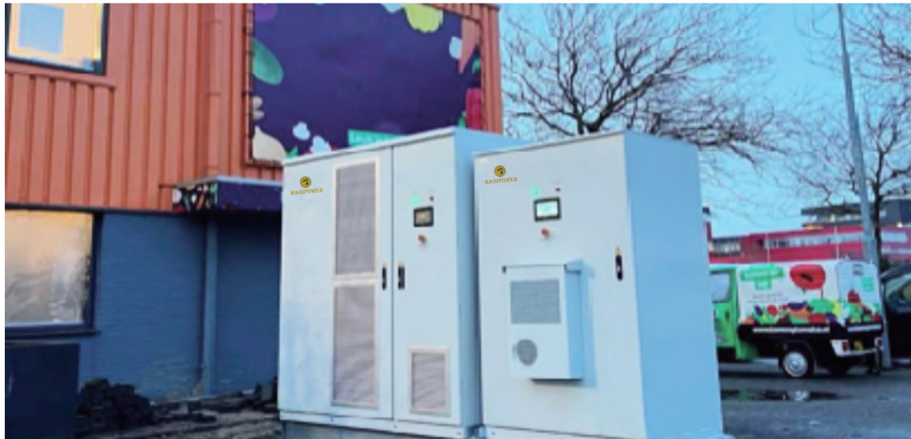
Netherlands · Backup Power Storage System for Steel Manufacturing Plant Scale:500kW / 860kWh
