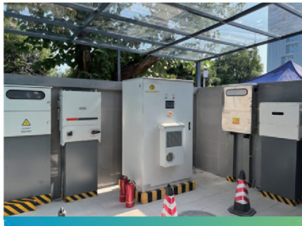
Sichuan · CNPC EV Solar-Storage-Charging Project Scale:100kW / 215kWh
