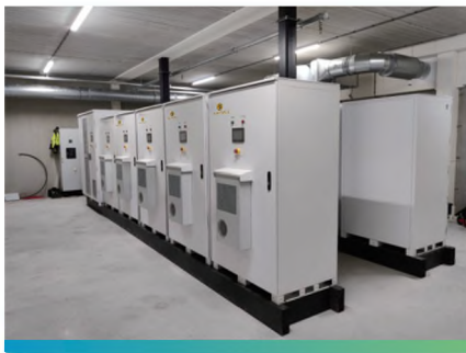
Netherlands · Large-Scale Camping Equipment Warehouse PV-Storage Project Scale:1MW / 2.15MWh
