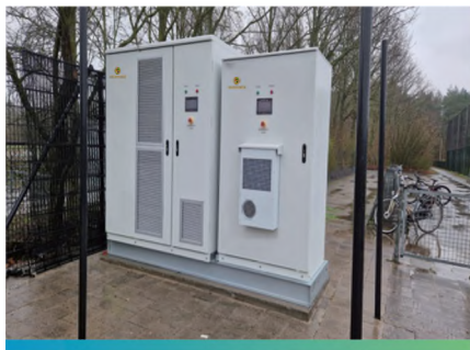
Netherlands · Livestock Farm Solar-Plus-Storage Installation Scale:62.5kW / 215kWh
