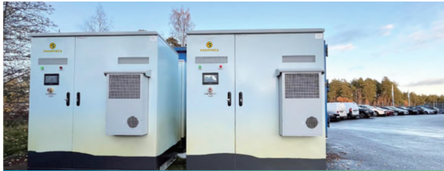
Sweden · Electric Vehicle Storage-Charging Project Scale:360kW / 633.6kWh
