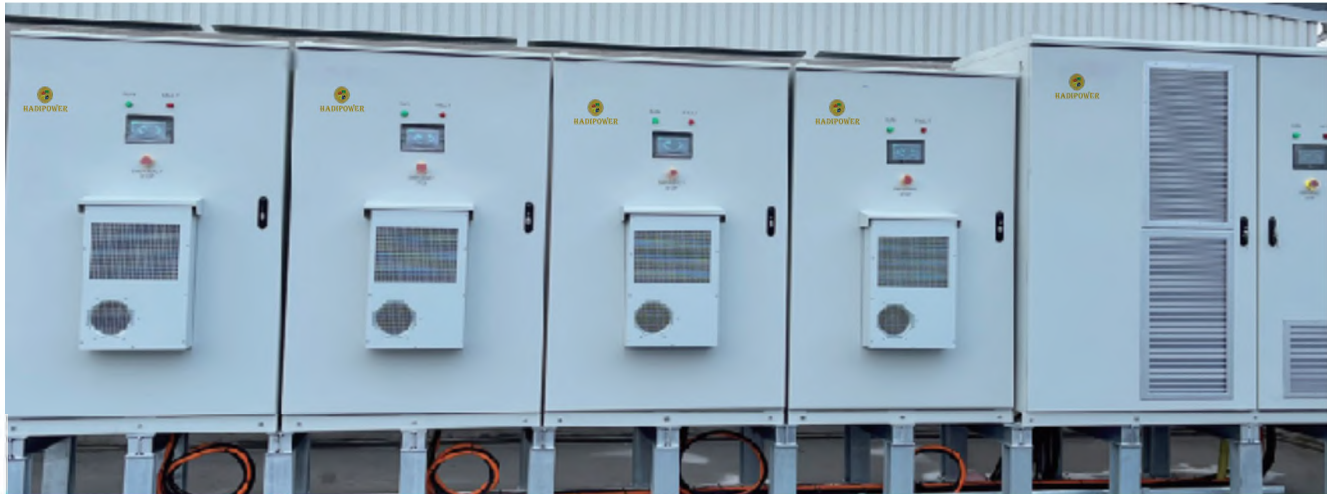
Netherlands · Backup Power Storage System for Catering Company Scale:125kW / 215kWh
